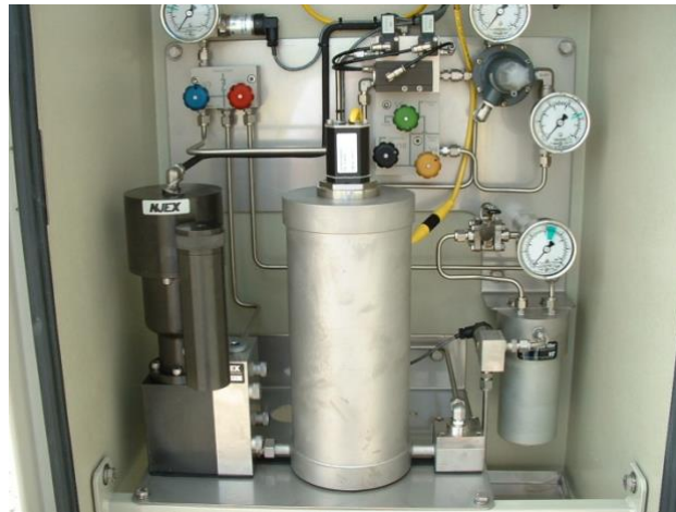
Figure 2; Injection Pump and Meter
