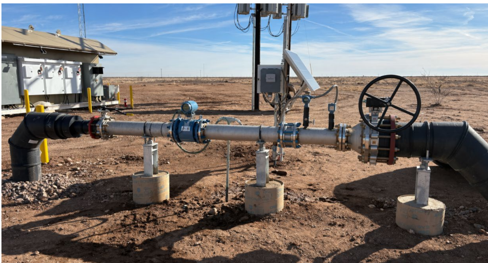
Figure 3. Example of proper mag meter installation
