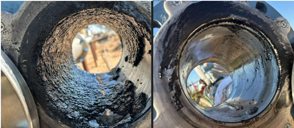
Figure 8. Meter condition before and after surface treatment
