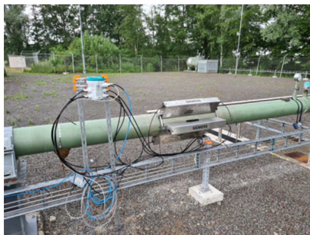
Figure 10. Four Beam, Weld Seal Transducer Installation
