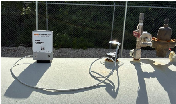
Figure 5: Watchtower Installed on 500 gal Bulk Tank
