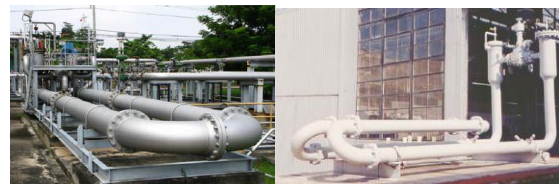
Figure 7: Examples of Pipe/Ball Provers
