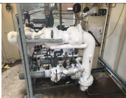
Figure 22: "Minor" freezing regulation station
