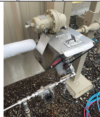
Figure 20: Enclosure Heater with frosted pipe
