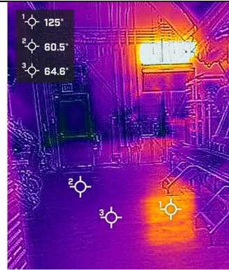
Figure 16: Thermal images showing 60F increase from unheated area
