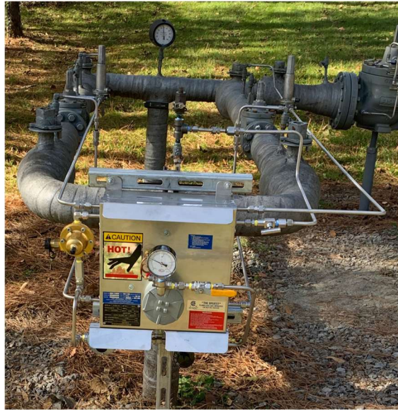
Figure 1: example pilot gas heater installation
