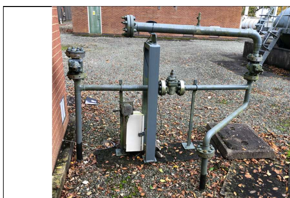
Figure 21: Regulation station with "minor freezing" problem
