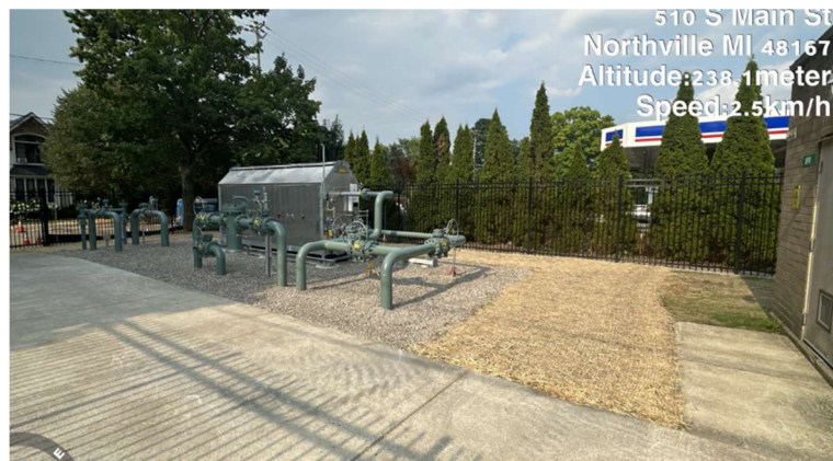
Figure 26: Large catalytic heater (500K+ BTU) installed next to gas station and across from houses
