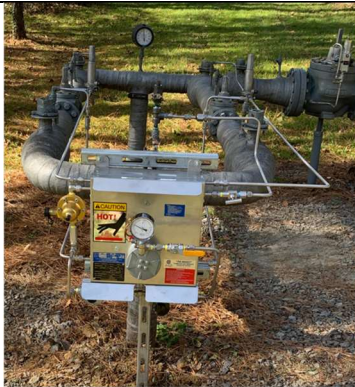
Figure 17: Pilot gas heating for two pilot regulators
