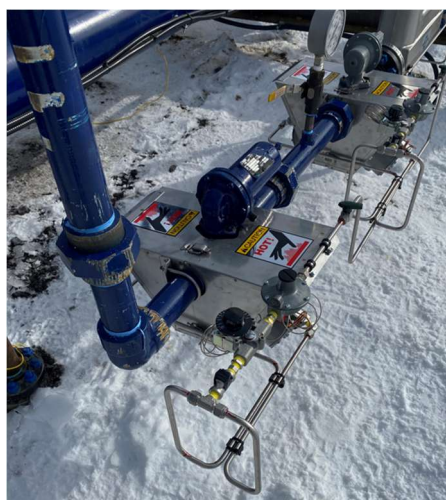
Figure 12: Example enclosure heater on a regulator; gas train shown with temperature controller
