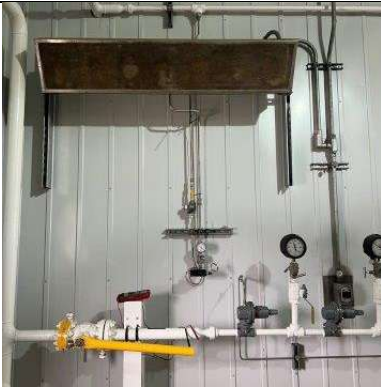
Figure 15: Catalytic heater in spacing heating application
