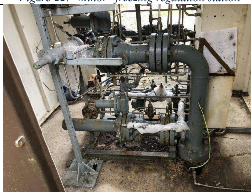
Figure 24: Regulation station after heaters installed, achieved 41F actual versus 35F estimated
