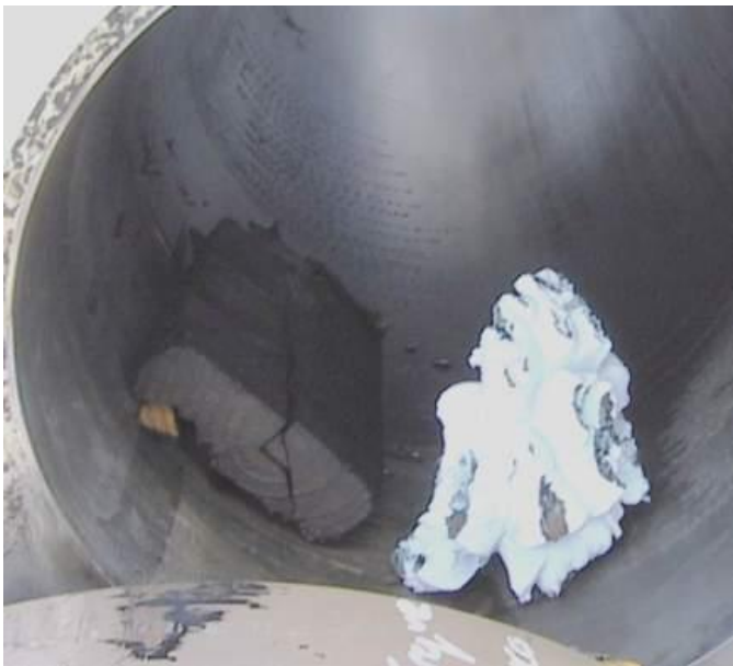
Figure 18 – 12-inch Flow Conditioner Blockage
