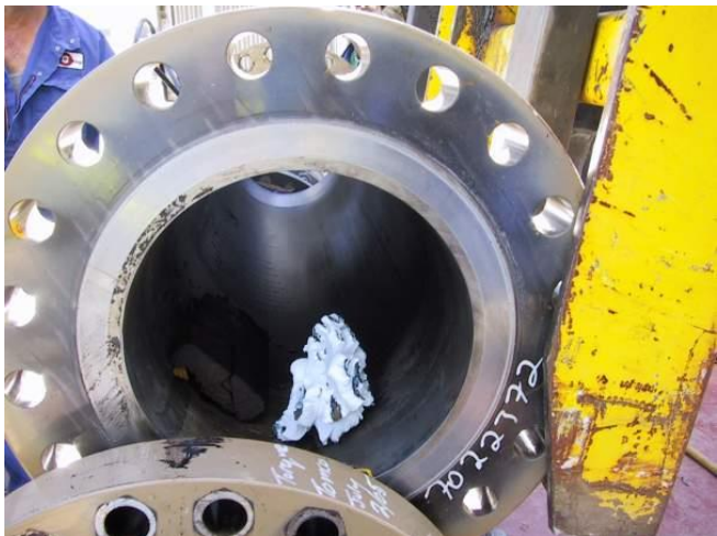
Figure 17 – 12-inch Flow Conditioner Blockage
