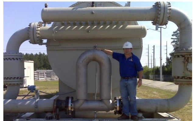
200mm (8") Coriolis meter installed in 250mm (12") line
