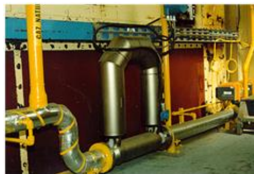
Combustion control application to boilers
