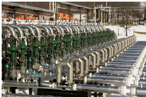
Coriolis Natural Gas Storage Measurement in Hungary
