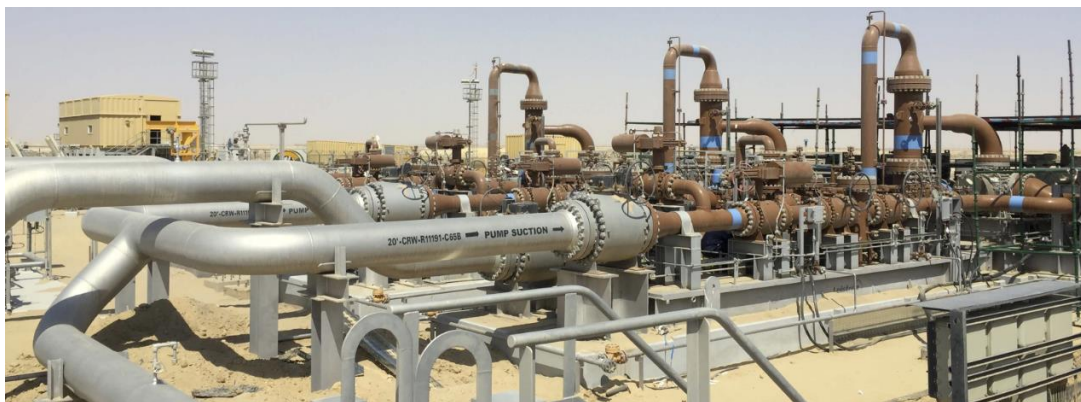
Figure 1. Gathering station where multiple oil and gas streams are combined and processed.
