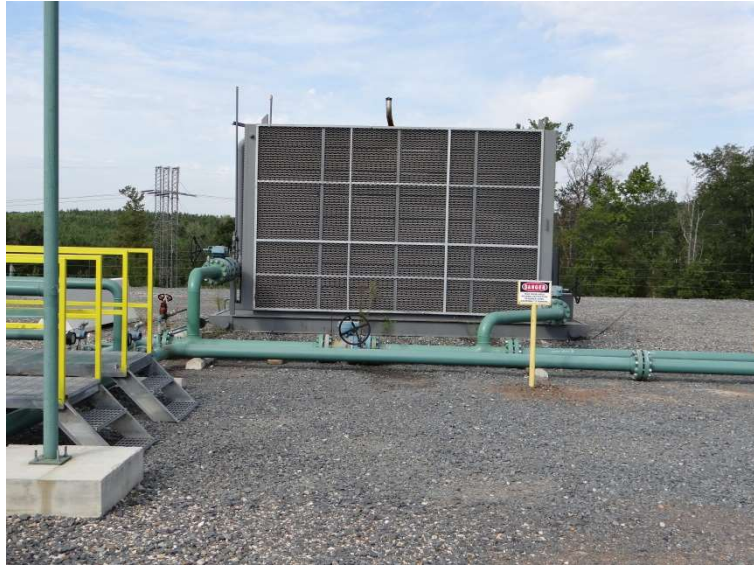
Figure 8: Heat Exchanger Keeps Average Temperature Within Operational Limits
