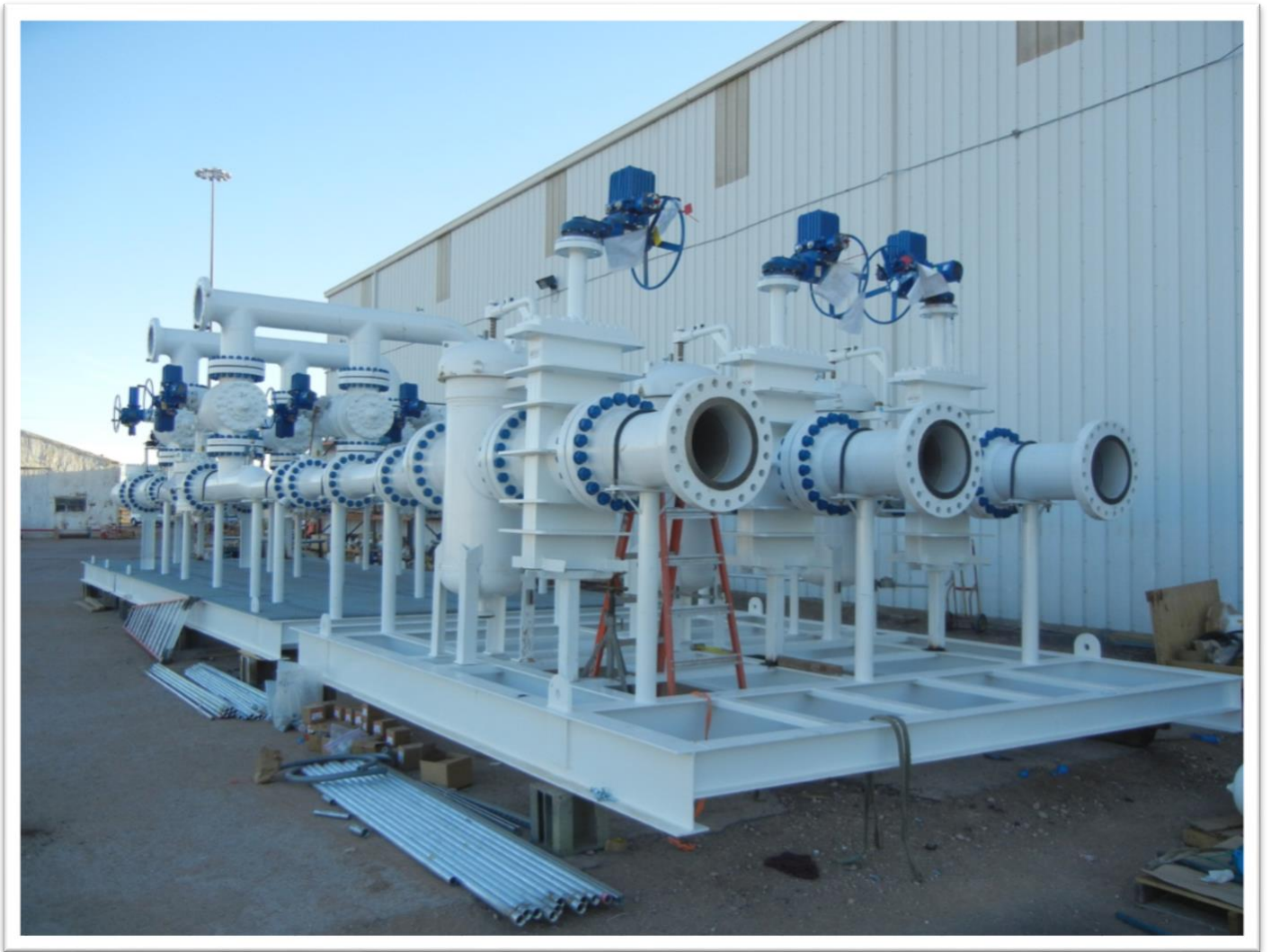
Figure 2 – Triple Turbine Meter Measurement Station
