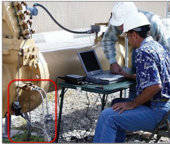
Figure 12. Example Square Root Error Pressure Transducer Installation (Photograph provided courtesy of PGI Division, Parker Hannifin Corporation)
