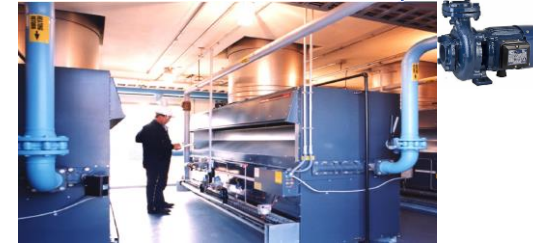
REMOTE GLYCOL WATER HEAT AND PUMP.
