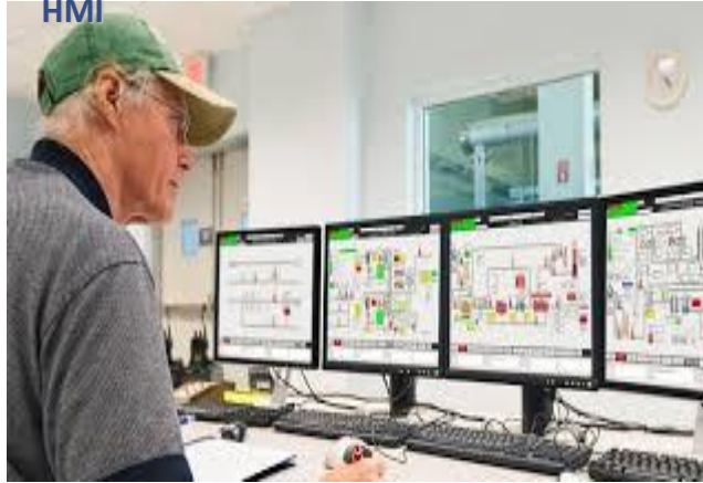
CONTROL CENTER 1 COMPUTERS AND HMI
