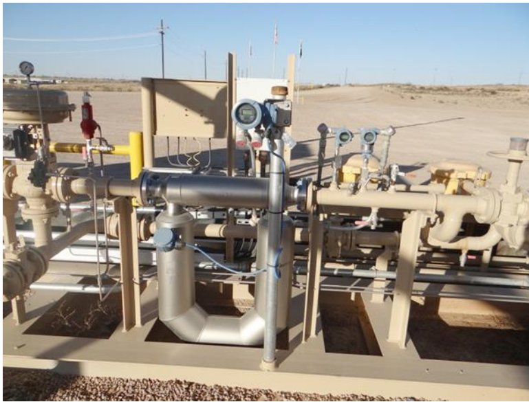
FIGURE 6: CORIOLIS METERS ARE COMMONLY USED
