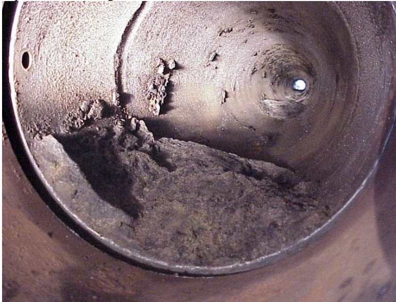
Figure 2. Contamination Buildup at the Plate Seat of an Orifice Flow Meter
