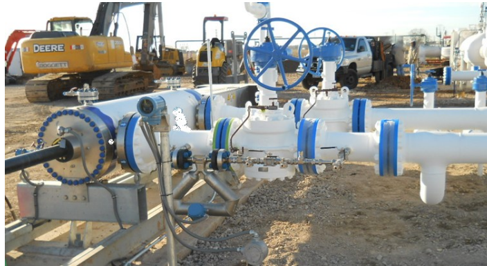
Figure 15 – Inferred Prover Installation
