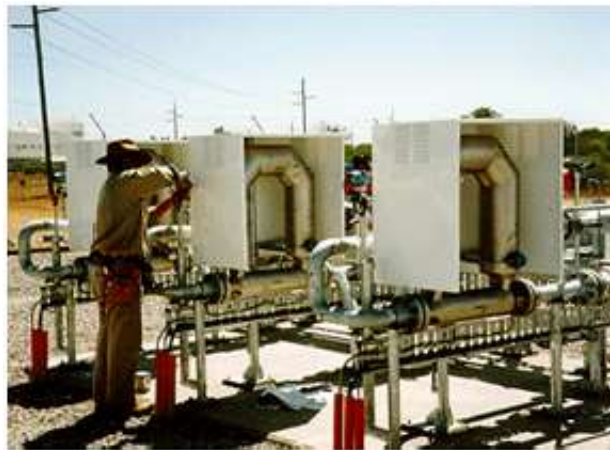
“After” installation since 1996, with two operating and one “hot spare” meter for 80:1 turndown.
