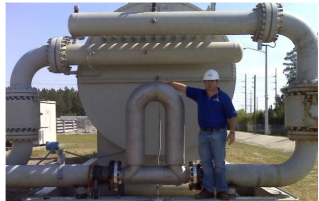
200mm (8") Coriolis meter installed in 250mm (12") line
