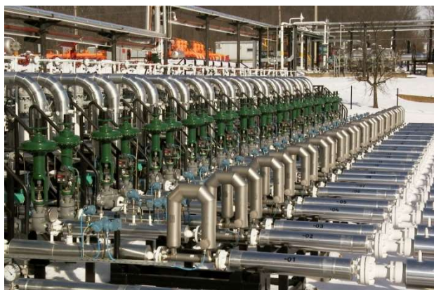
Coriolis Natural Gas Storage Measurement in Hungary
