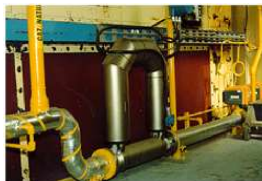
Combustion control application to boilers
