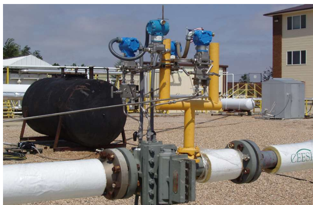
FIGURE 6. 4", Orifice Meter Under Wet Gas Flow Testing
