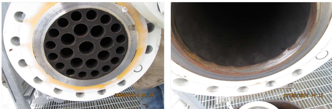
Figure 2. Measurement Accuracy Improvements Resulting from Meter Tube and Flow Conditioner Cleaning
