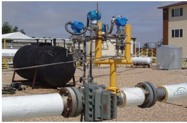
FIGURE 6. 4" orifice meter under wet gas flow testing
