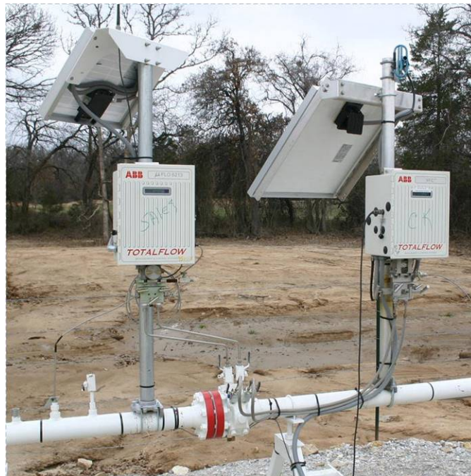
Figure 1. Example Orifice Check Flow Meter Installation with Redundant Pressure Taps, Pressure Transmitters, and Electronic Gas Measurement
