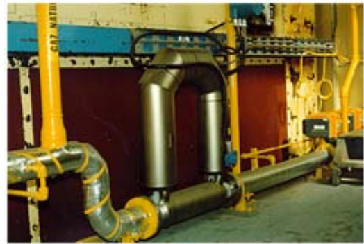
Combustion control application to boilers
