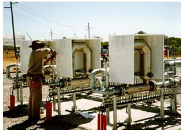
“After” installation since 1996, with two operating and one “hot spare” meter for 80:1 turndown.
