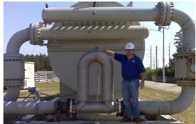
200mm (8") Coriolis meter installed in 250mm (12") line
