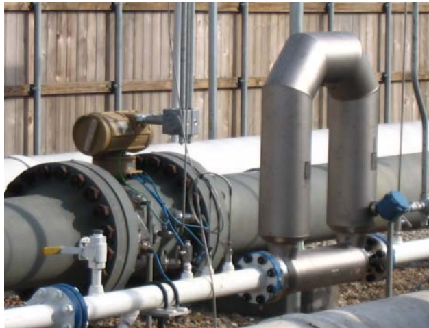
Parallel 3" Coriolis and 16" ultrasonic in a fuel gas metering installation.
