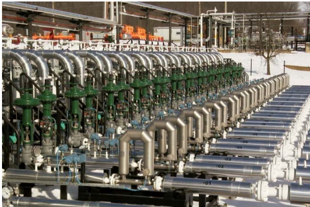
Coriolis Natural Gas Storage Measurement in Hungary
