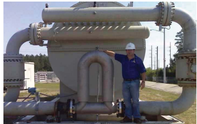
200mm (8") Coriolis meter installed in 250mm (12") line
