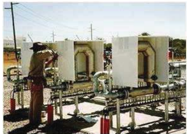
"After" installation since 1996, with two operating and one "hot spare" meter for 80:1 turndown.
