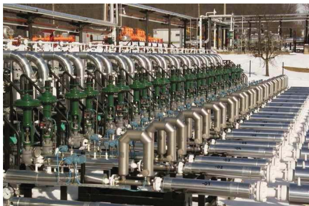
Coriolis Natural Gas Storage Measurement in Hungary
