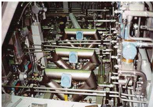
Coriolis Fuel Gas Measurement on a Gas Turbine
