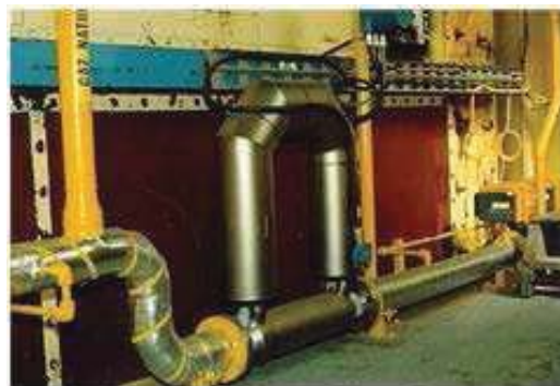
Combustion control application to boilers
