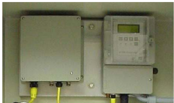
Figure 2; Injection Rate Controller
