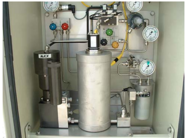
Figure 2; Injection Pump and Meter
