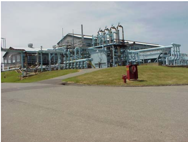
Figure 2. Rockville Peak Shaving Plant
