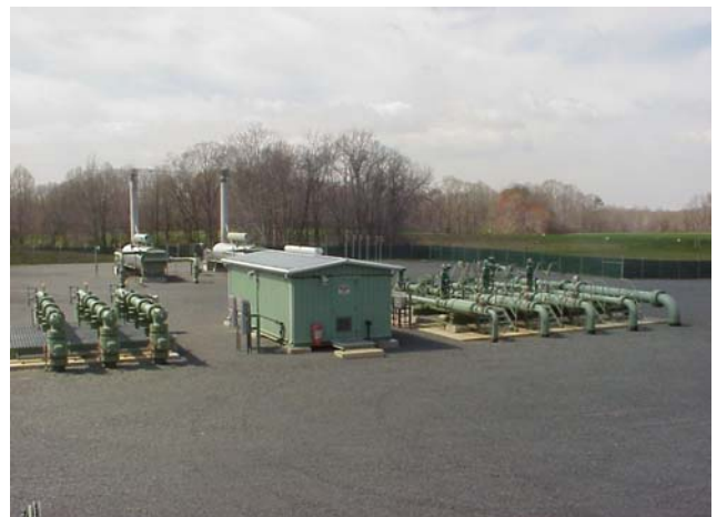
Figure 1. Gardiner Road Gate Station
