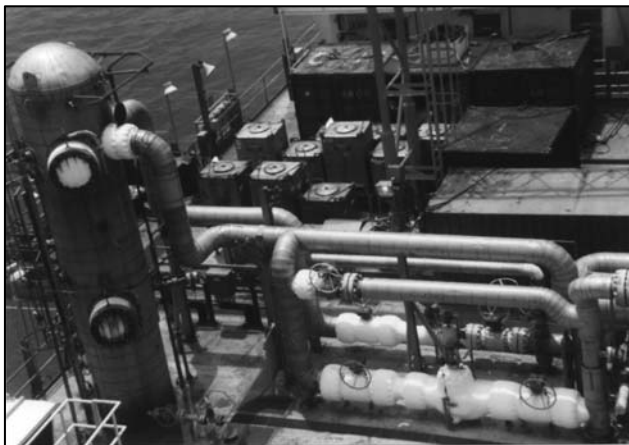
Figure 3: Hydrocarbon dew point reduction plant
