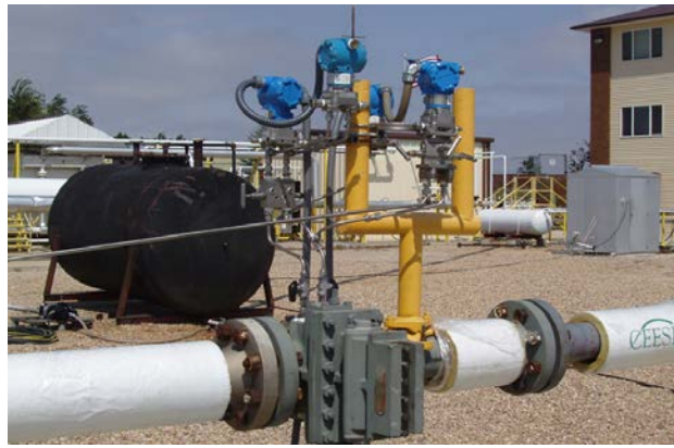
FIGURE 6. 4" orifice meter under wet gas flow testing
