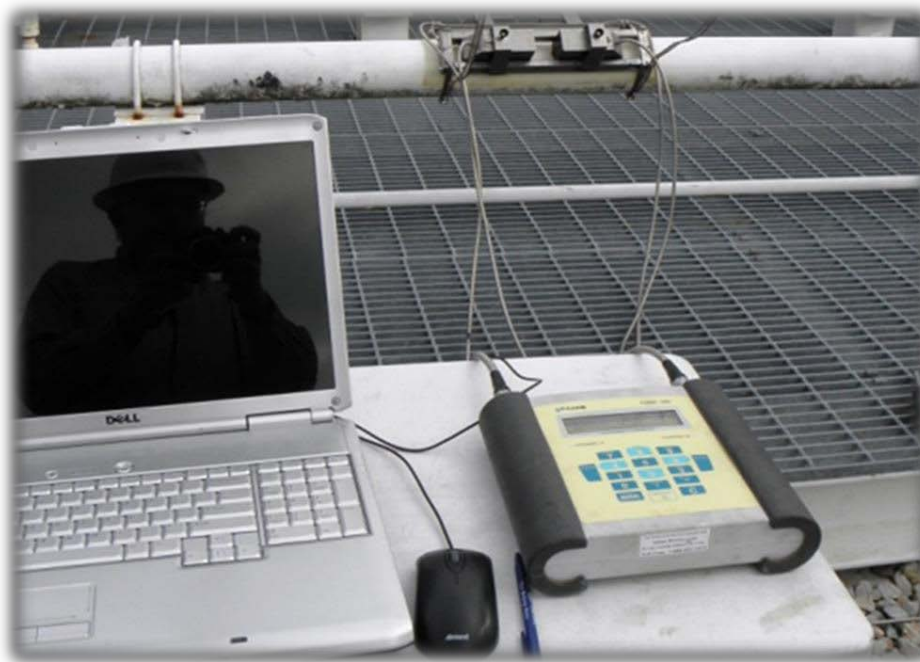
Figure IV. - CLAMP-ON METER INSTALLED ON PIPE
