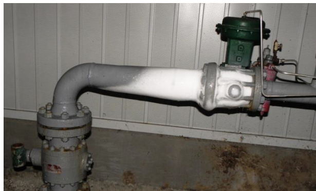
Figure XIV. - ICE IS CERTAIN LEAKAGE EVIDENCE
