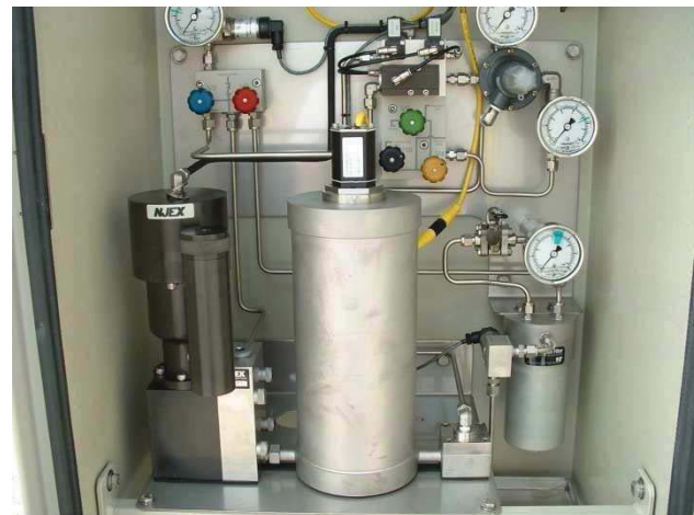
Figure 2; Injection Pump and Meter
