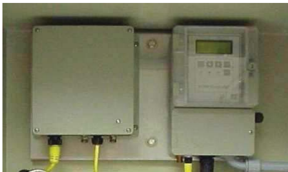
Figure 3; Injection Rate Controller
